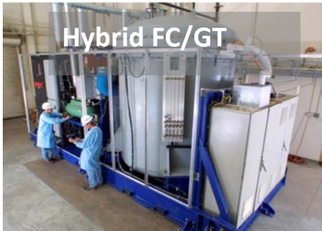
World first SOFC-GT system
